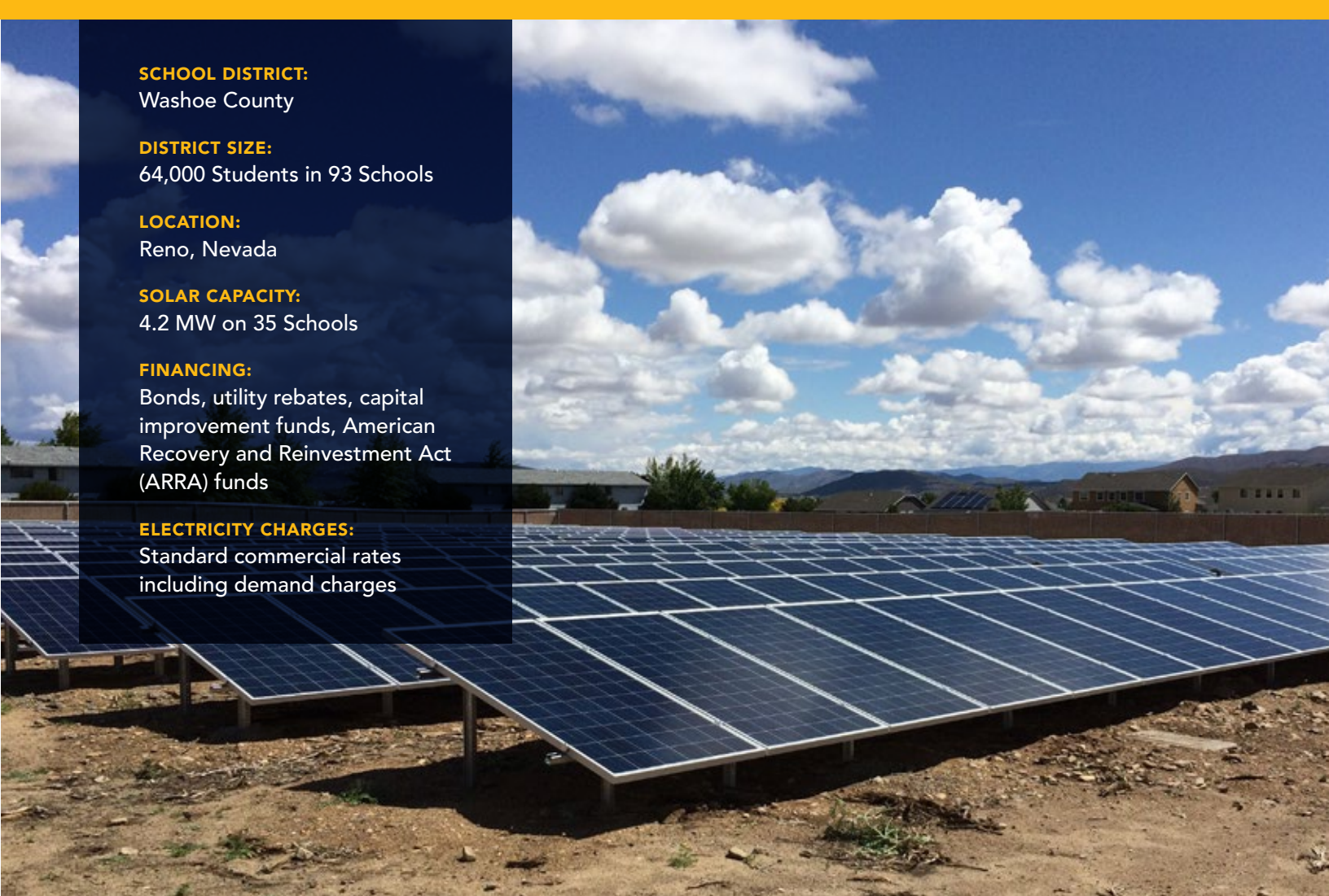
Stead Elementary School's 125 kW array allows 100% of savings to stay at this Title I school.
