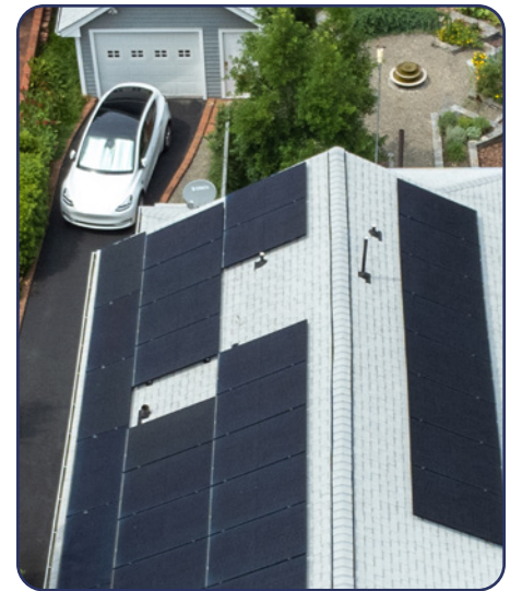
1 DAVID'S HOME SOLAR AND EV
